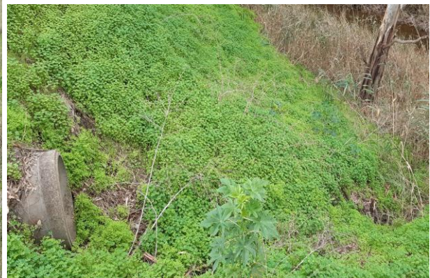
Outlet to river. No flood flap
