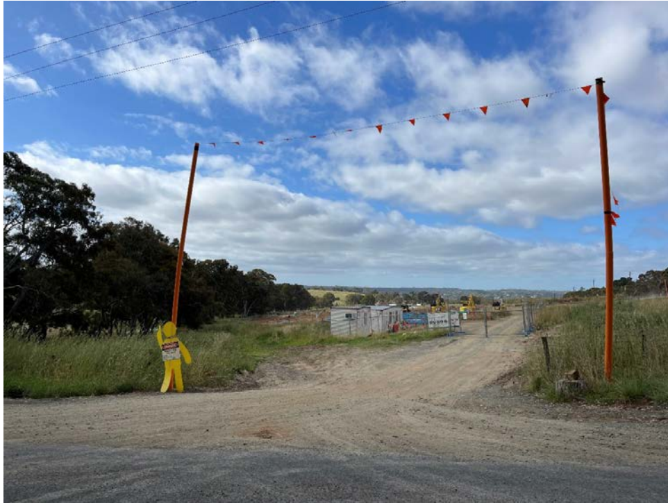
'Glen Lea' housing development, where all the magnificent Red Gums and Blue Gums, except those in the winter creek line, have already been destroyed and removal of topsoil is underway.
