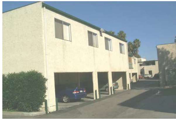
Figure A1-03 - Example of soft storey conditions, where parking requirements result in large weak openings.
