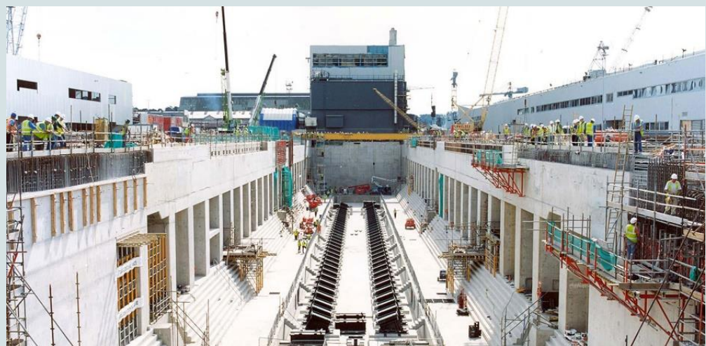
Figure 2.10 - Photo showing 9 Dock at Devonport in the United Kingdom (Source: Navy Lookout 2020)
