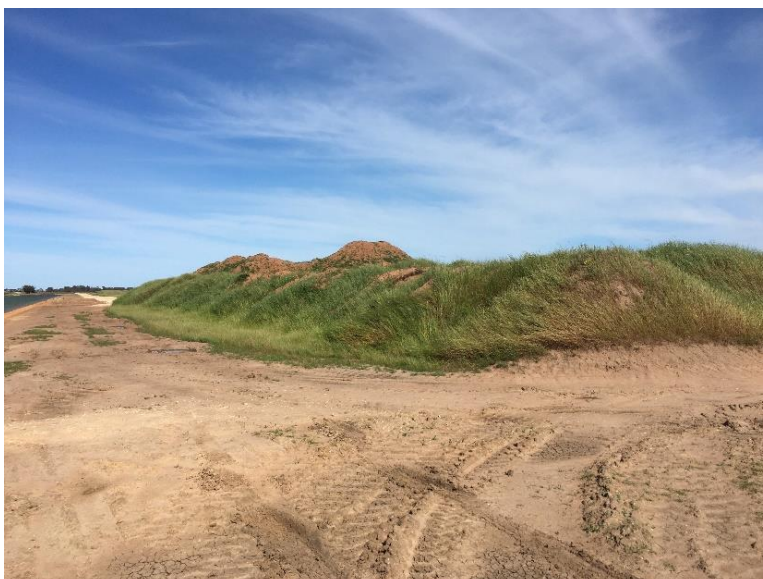
Photograph 13. Stockpiles of topsoil from excavation of stormwater detention channel at southern site boundary. 17.10.2022.
