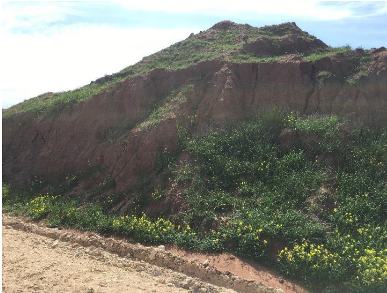
Photograph 14. Stockpile of topsoil from excavation of stormwater detention channel at southern site boundary. 17.10.2022.
