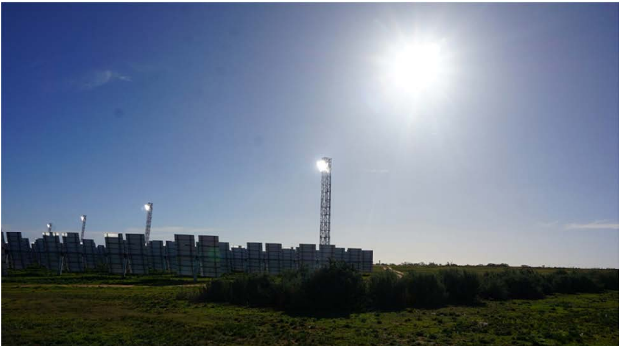
Figure 33 - Photograph of all four solar receiver towers and heliostat fields in operation at Carwarp demonstration facility, Victoria.
