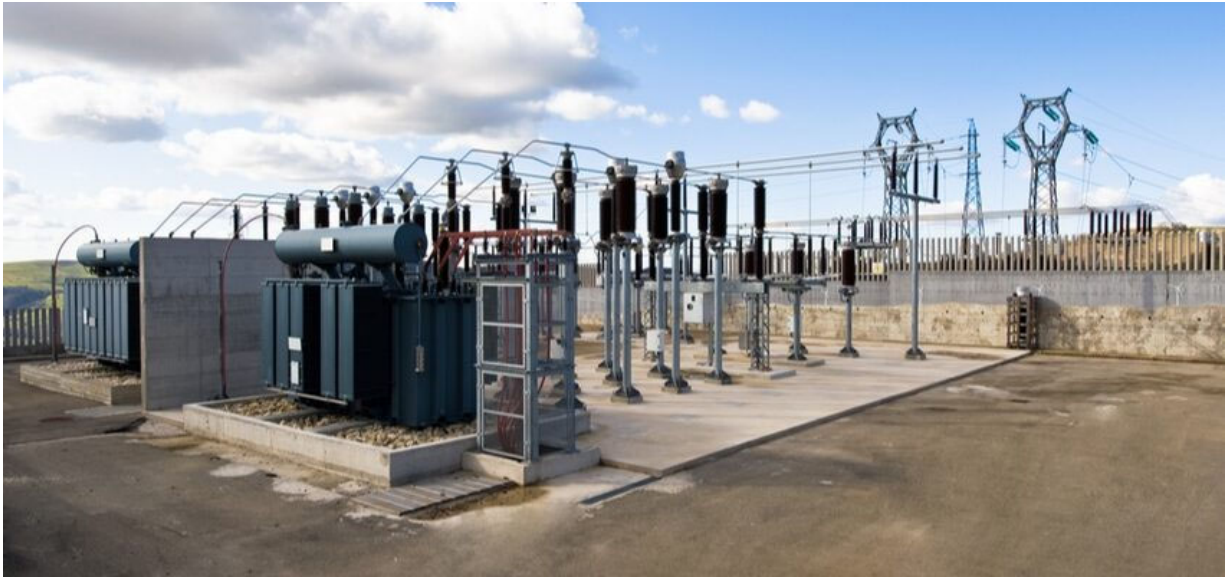
Figure 25: Photograph of a typical substation
