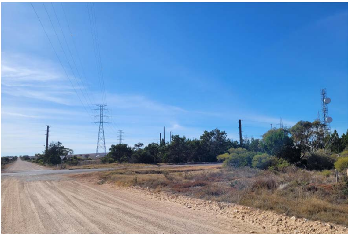
Figure 3: View of Yadnarie substation infrastructure and 132kV transmission line as viewed from Pine Corner Road, across Birdseye Highway in a northerly direction.
