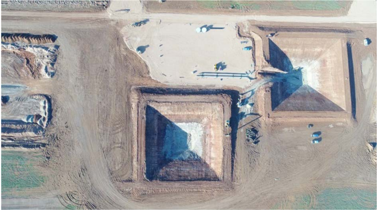
Figure 22: Thermal Hydro pits, during construction at RayGen’s commercial demonstration facility - Carwarp, Victoria.
