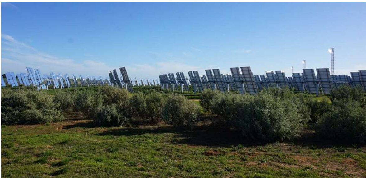
Figure 1: RayGen technology operating at Carwarp, Victoria
