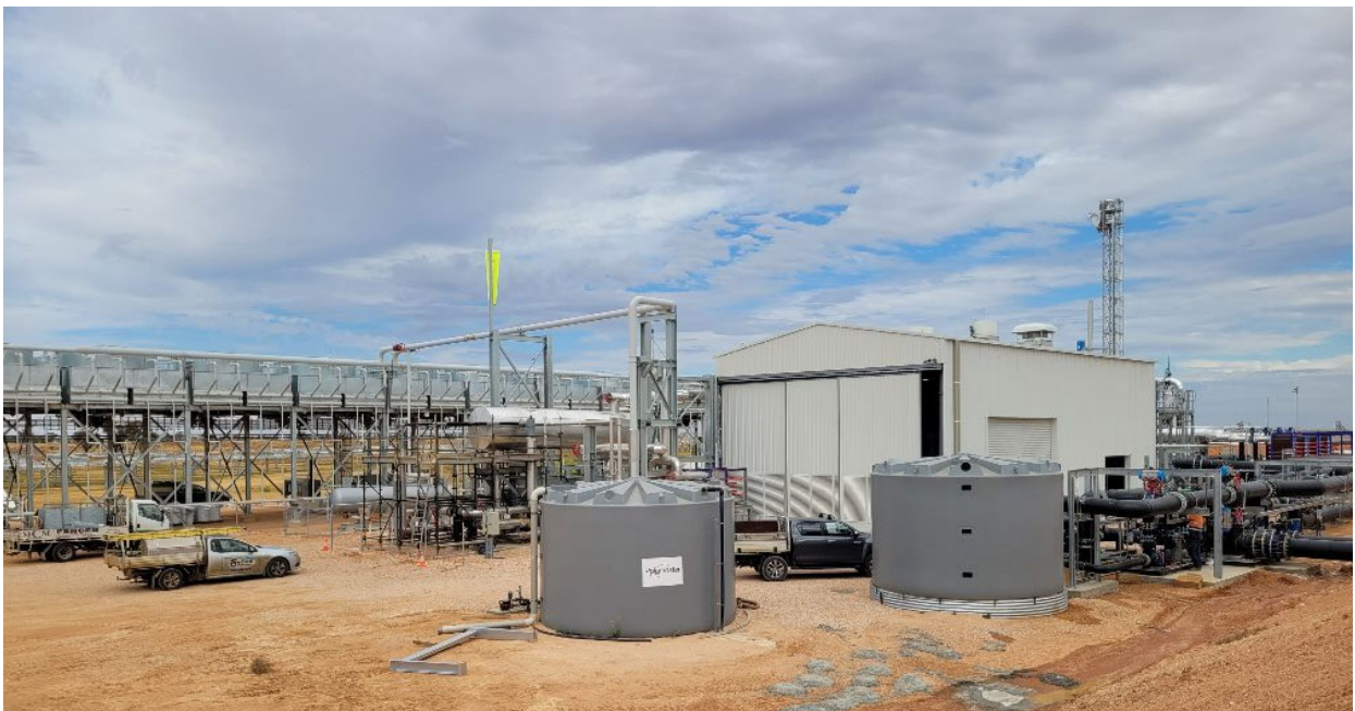
Figure 9: Thermal Hydro plant and equipment - RayGen site - Carwarp, Victoria.
