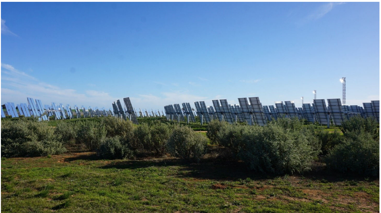
Figure 7: Photograph of heliostats and receiver at RayGen site - Carwarp, Victoria.
