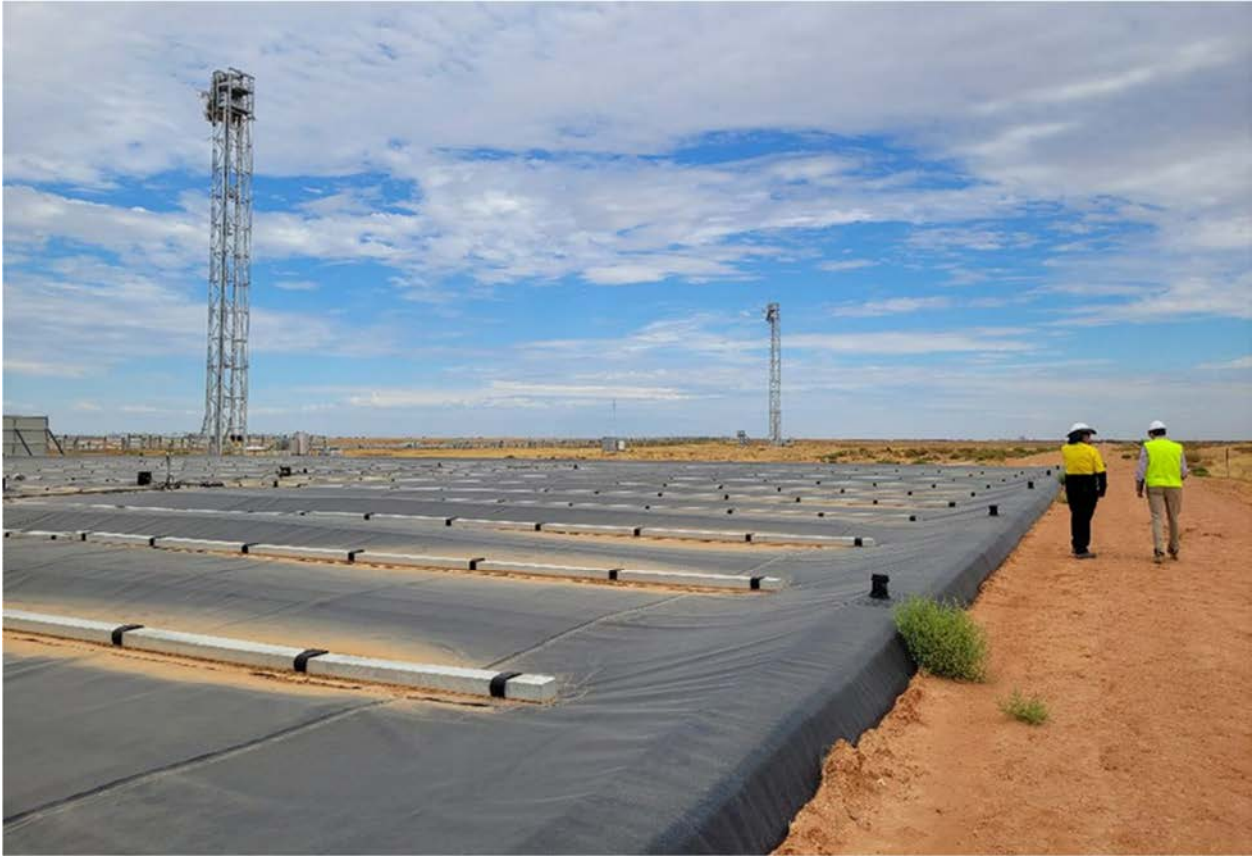
Figure 8: Thermal Hydro pit and receiver at RayGen site - Carwarp, Victoria.
