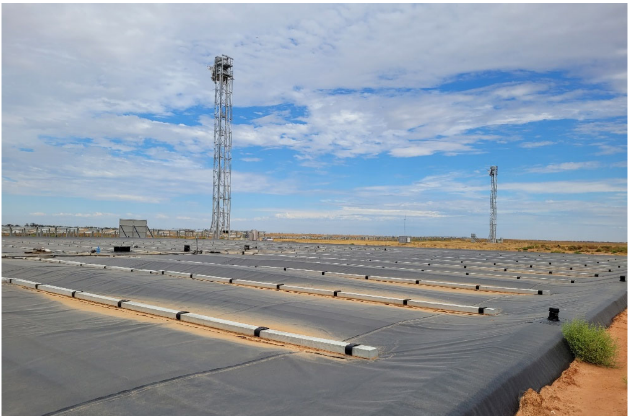
Figure 23: Photograph of a Thermal Hydro pit and receiver at RayGen demonstration facility - Carwarp, Victoria.
