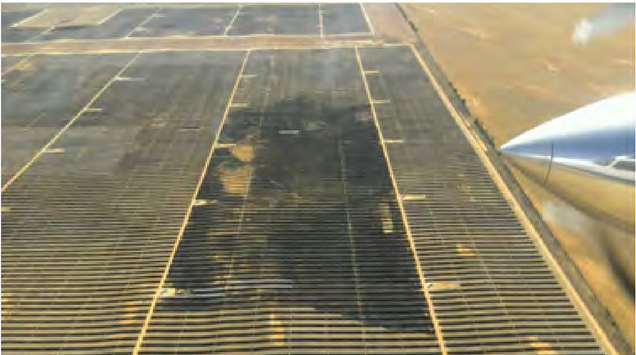
CFA air response to a grass fire in a solar facility, December 2022.
