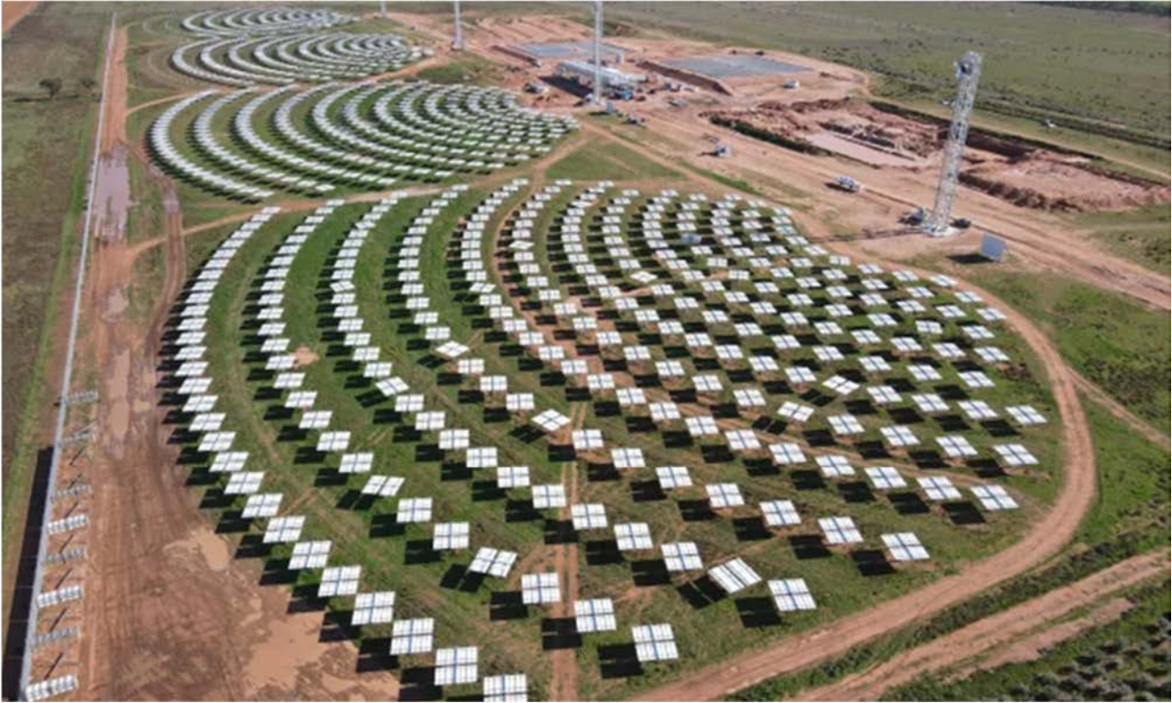
Figure 2: RayGen commercial demonstration facility Carwarp, Victoria – Source photograph RayGen
