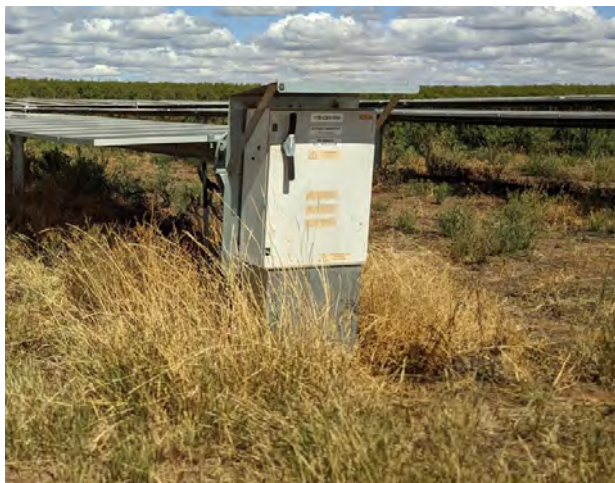
Unmanaged vegetation at string commander box.
