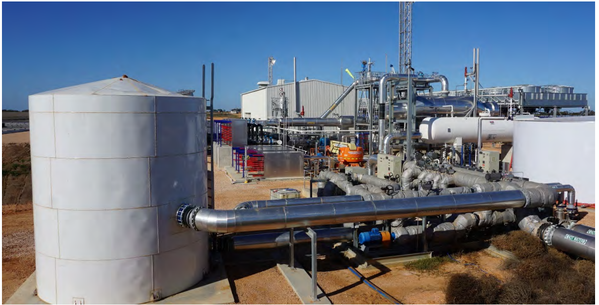
Figure 3: Typical power block at the Carwarp Facility, Victoria
