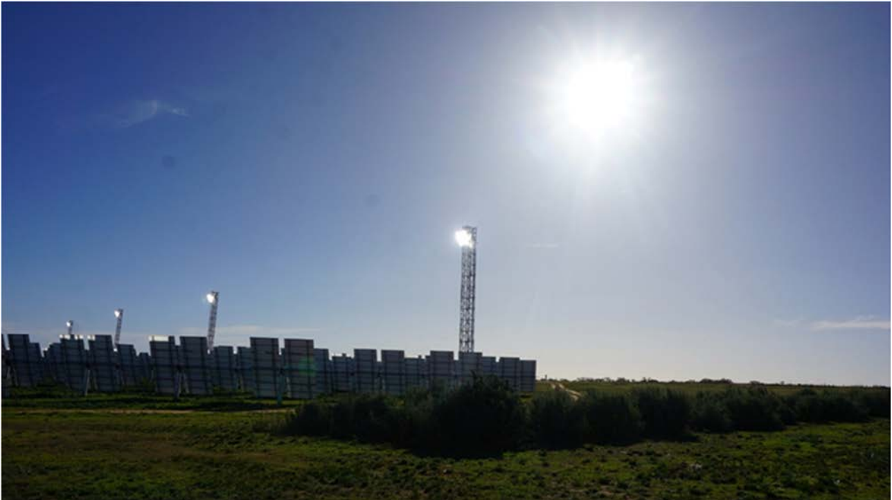
Figure 9: Photograph of all four solar receiving tower and heliostats in operation at Carwarp demonstration facility, Victoria.
