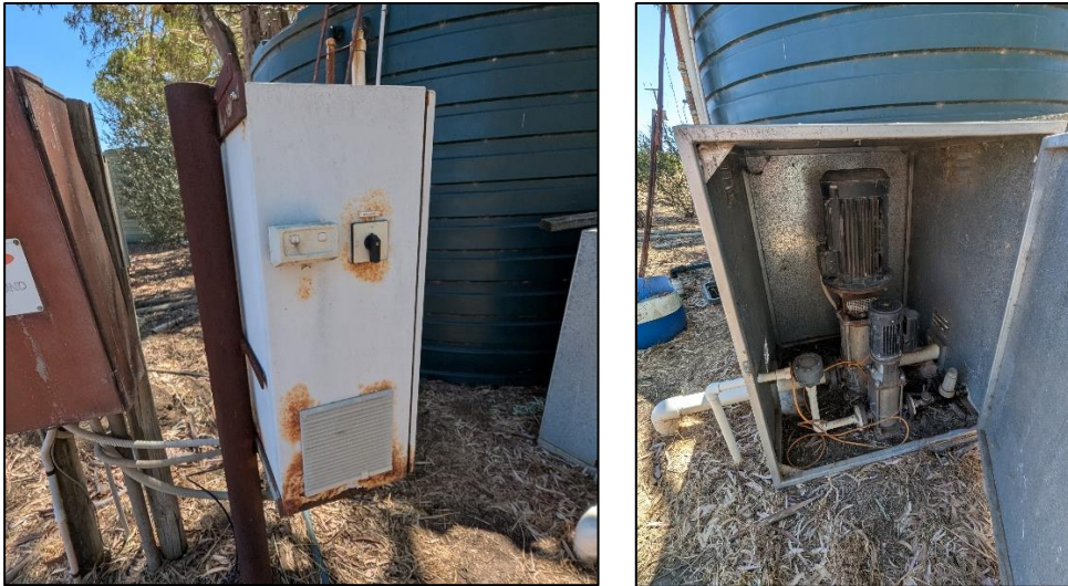
Existing privately owned groundwater infrastructure and pumpset
