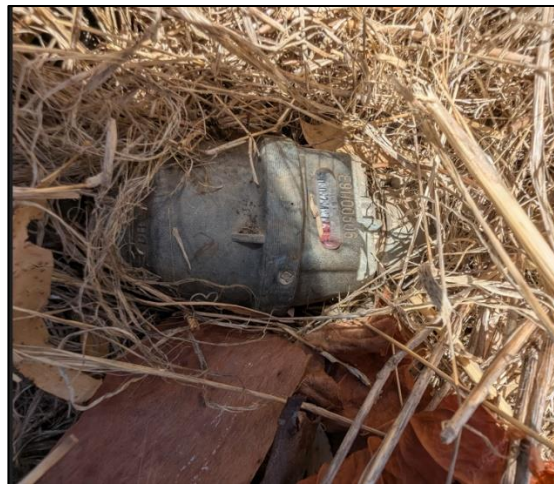
Existing Ø20mm water meter connection located on Hoffnungsthal Road (ID: E91100506)
