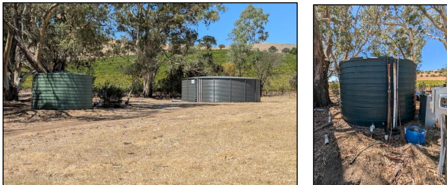
Existing onsite groundwater holding tanks
