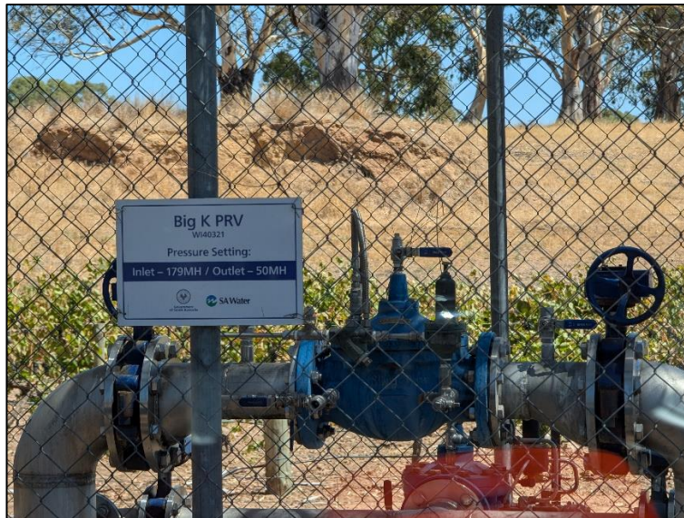
Existing PRV station located on intersection between SAWC water mains and transmission main
