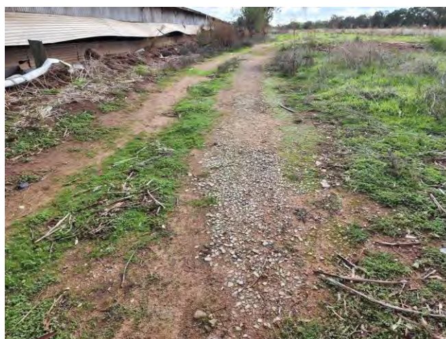
Item 1 – Driveway – Debris throughout
