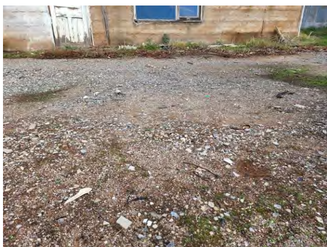
Item 1 – Driveway – Debris throughout
