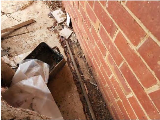
Item 5 – House, debris
