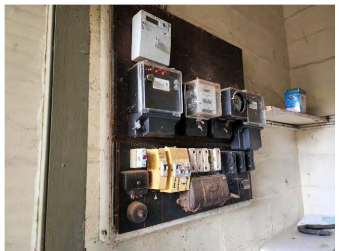
Item 6 – House, electrical board and switches
