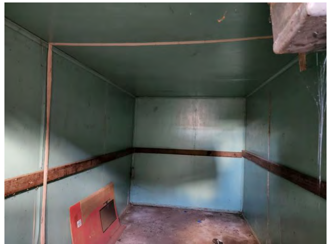
Item 8 – Storage container (internal)
